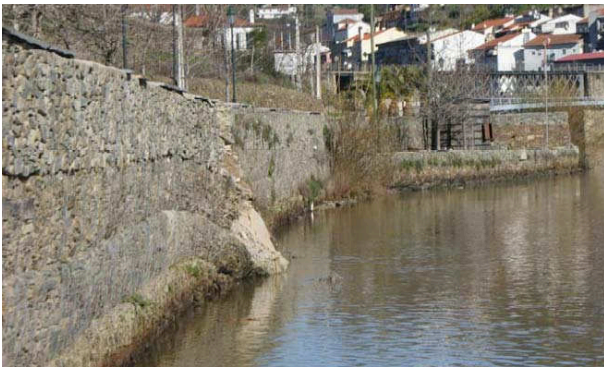
Fig. 5 Collapsed gabion wall
