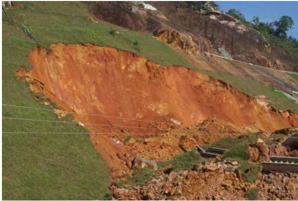
Fig. 2 After the catastrophic failure
