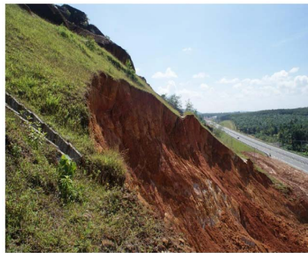
Fig. 3 Failure surface is shallow. Whitish clayey is seen at some locations
