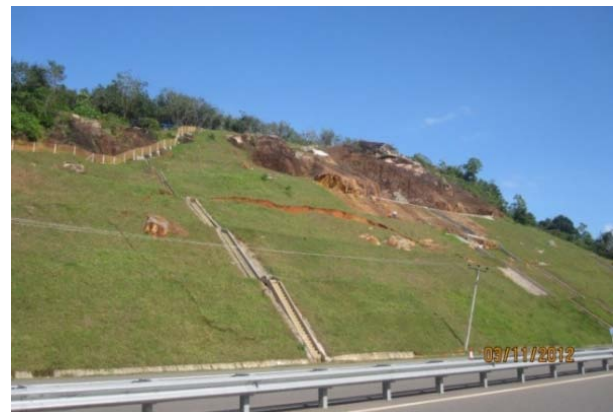
Fig. 1 Tension cracks on the verge of failure
