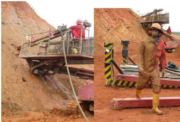
Fig. 8 Water oozing out of relict joints during drilling
