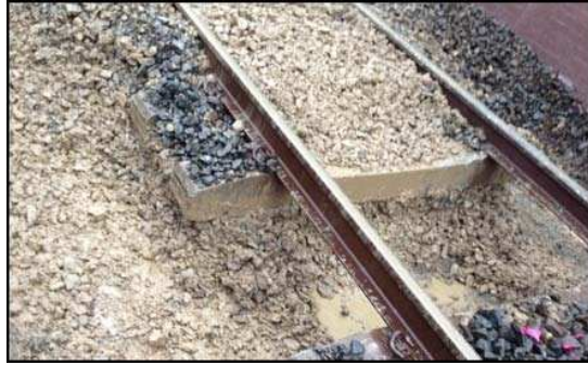
Fig. 2 Ballast fouling due to clay pumping (Photograph were taken during track maintenance at Ashfield, NSW).
