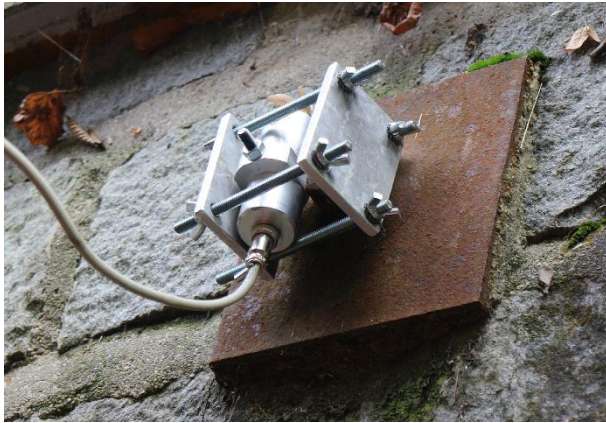
Figure 9. Force-fitted installation of the accelerometer sensor to conduct acoustic logging measurements.
