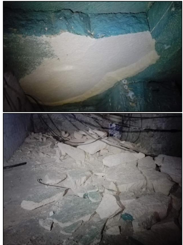
Figure 7. Failed roof of a cellar in Törökbálint (foto: P. Görög)
