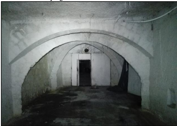
Figure 6. A photo of the rectangular cross-sectioned cellar with masonry arches (foto: P. Görög)
