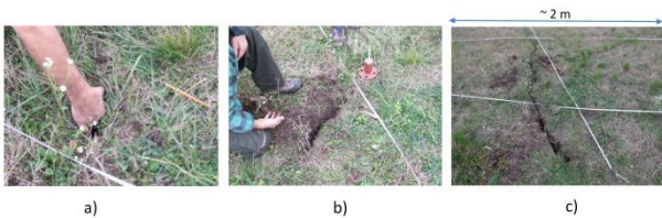
Figure 2. The exploration of cracks. a) Exploration of the crack detected by the Pre-P method and removal of vegetation; b) A partially explored crack; c) Part of the crack which has been excavated for longer distance.
