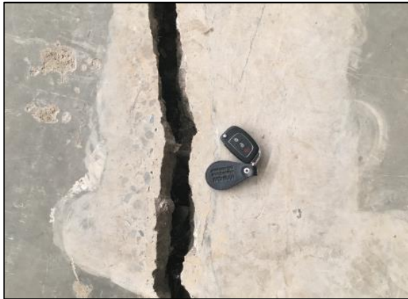
Figure 19. Fissures observed on the inside concrete floor.
