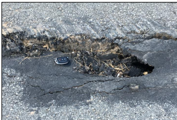
Figure 20. Displacements observed on the external asphalt pavement.
