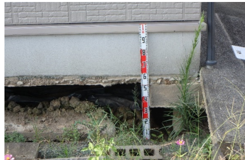
Figure 11. Exposure of pile-supported foundation due to liquefaction.
