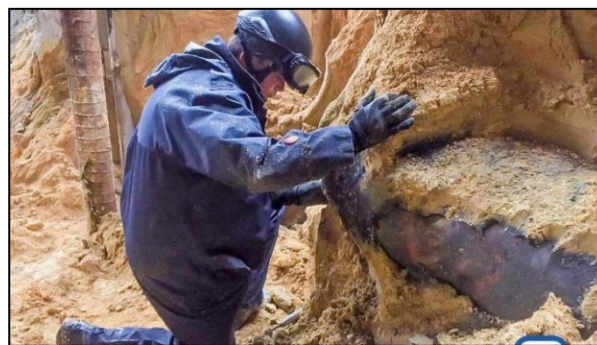
Figure 1. One of two WW2 x 1,000 lb AN-M65 bombs discovered on a waterfront construction site. January 2018, Convention Avenue, Wanchai (courtesy South China Morning Post)
