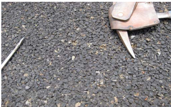
Figure 3. An example of poor quality basaltic cover (seal) aggregate exhibiting premature break down on a newly constructed pavement overlay. In this case, the count of moisture sensitive non-durable weak particles exceeds the specification limit.
