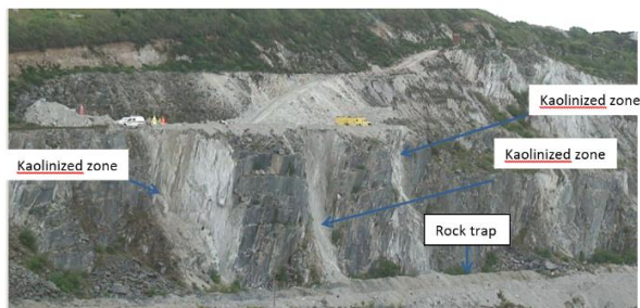
Figure 1. Photograph of a section of historical bench face (striking N-S) with several sub-vertical kaolinized zones, found within poorly kaolinized rock. Discontinuities sets of high angle joints striking sub parallel to the face subject to possible toppling failure.
