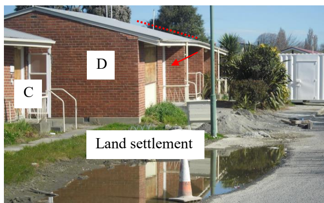
Figure 5 – Building D differential settlement (view roof line). Building ‘broken’ around dotted line.
