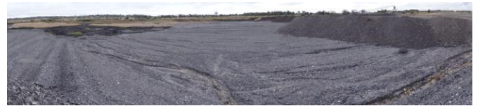
Figure 12. Progress of capping of TSF1 as at 25 June 2015, showing the initial 1 m thick layer and the follow-up 2 to 3 m thick layer of coarse reject.
