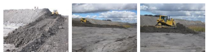
Figure 9. Early pushing of a capping of coarse reject over old bow-wave of surface TSF.
