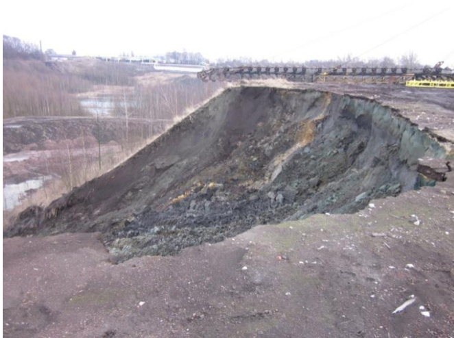
Figure 8. Photo of the unstable zone after sliding
