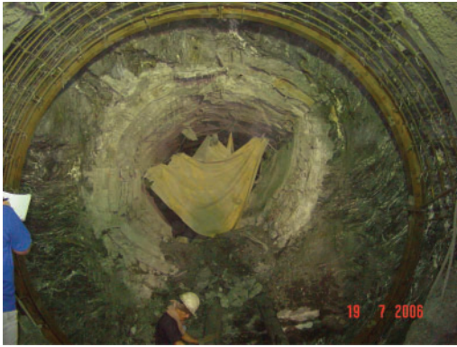
Figure 7. Large convergences at Yacambú-Quibor tunnel. (Courtesy of Ing. V. Camejo.)
