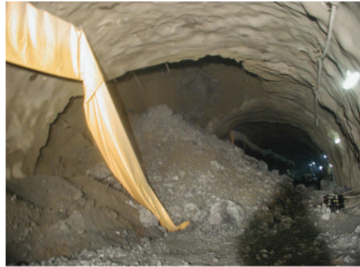
(a) Initial collapse
