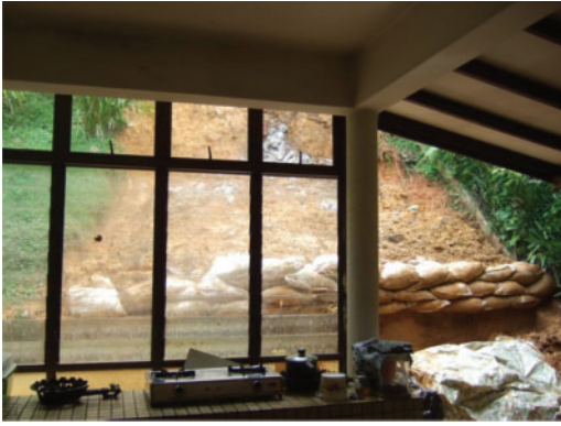
Figure 2. Photograph of landslide behind a house in Singapore.
