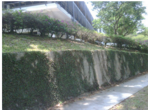
Figure 5. Photograph of blocked weep holes on a retaining wall taken by a student.
