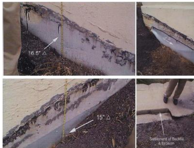
Fig. 5 Bridge approach slab settlement in Johnson County, Texas, USA
