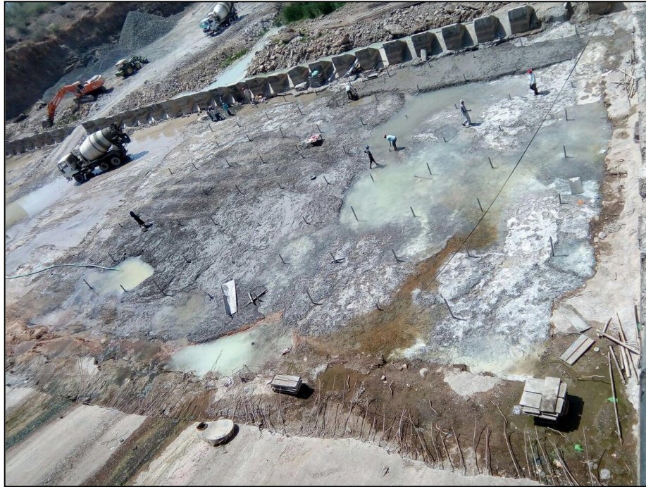
Photo – 2 Top View of Pulled Out Reinforcement at Toe and Damaged Apron
