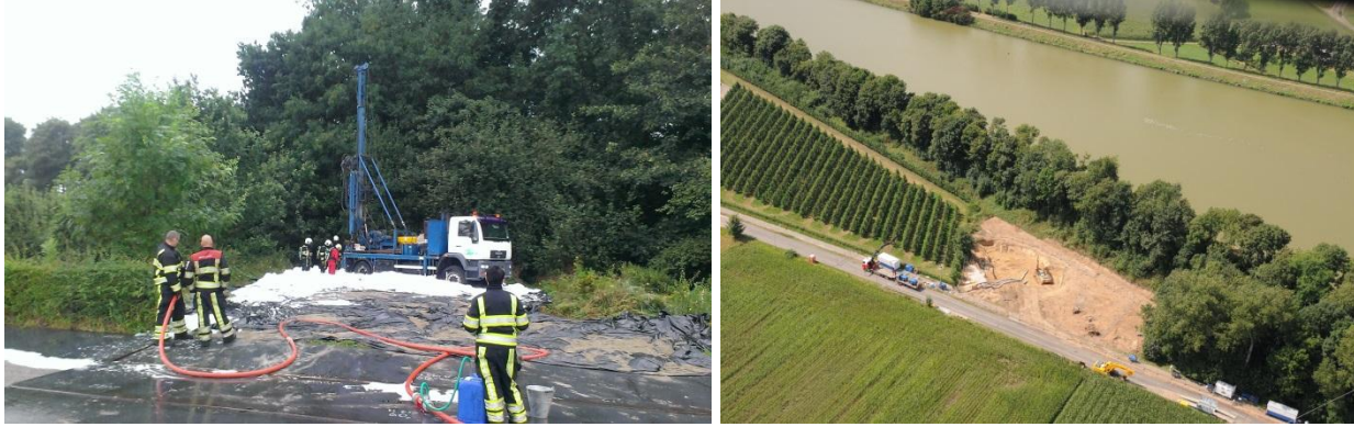
Figure 4. Location of the incident showing the drilling rig and the brushwood (left) and an aerial overview after clearing during refilling (right)
