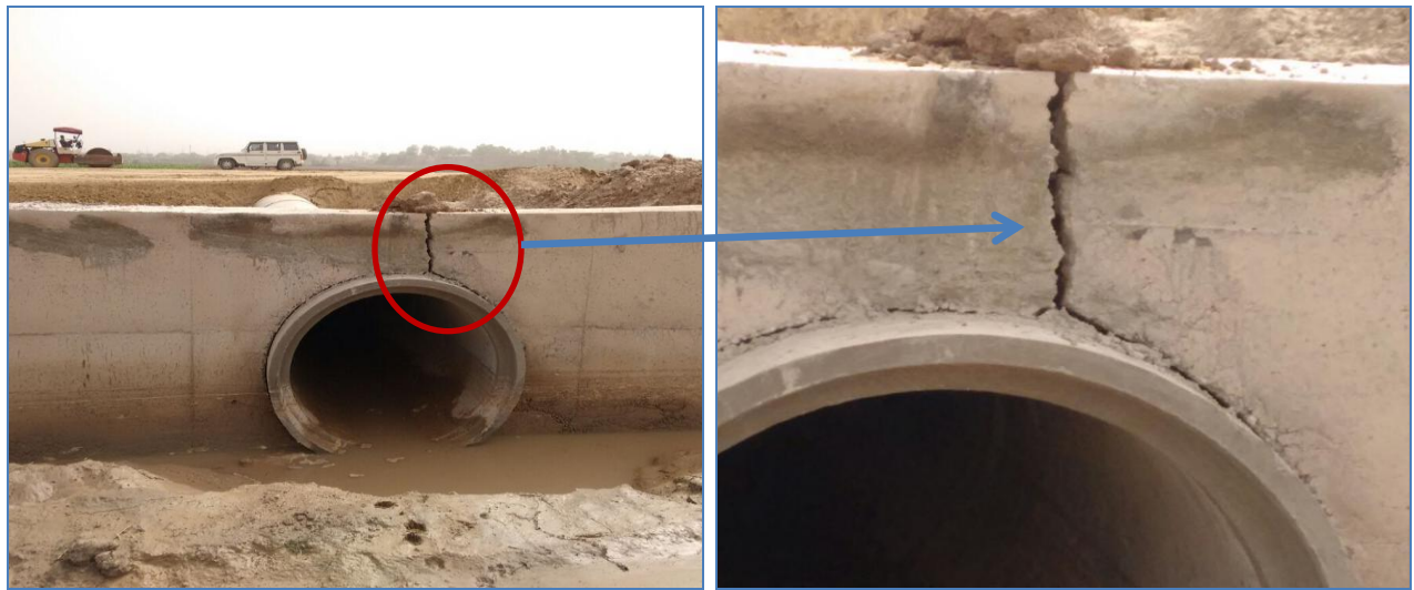
Figure 2 Crack development in the head wall of a typical Hume pipe culvert
