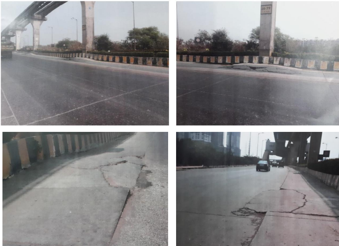
Figure 1: Pavement distress along Wadala-Sewri highway
