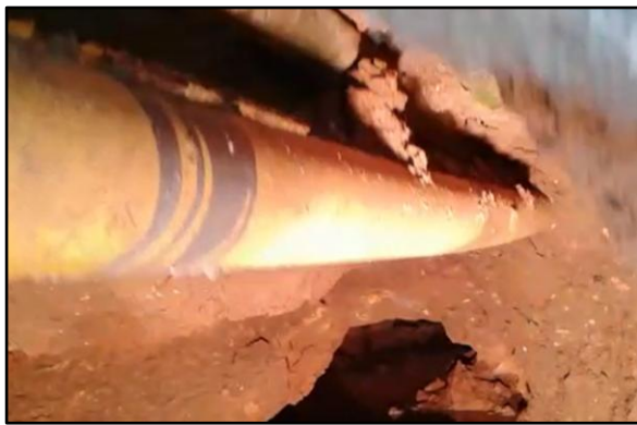
Figure 5. Utilities and water in the other underground cavity.
