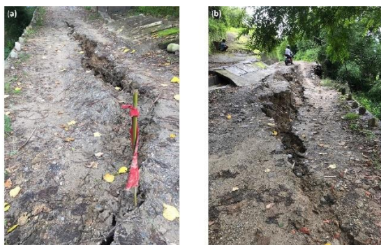
Figure 5. Cracks formed in road adjacent to Pyarienii jhora (a) on 27 th July, 2020 and (b) on 6 th August, 2020
