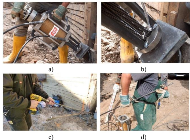
Figure 15. Anchor removal steps of DYWIDAG QuickEx: a) Detensioning strands with light jack; b) Wedge removal with magnetized tool; c) Rotating strand with hand drill; d) Extracting strand by hand (Bogdan and Wörle, 2018).
