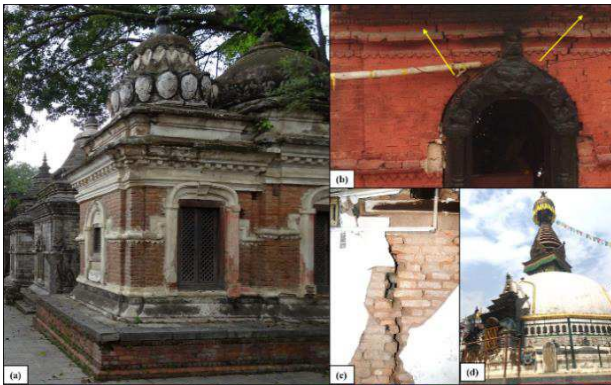
Figure 7. Temple structures common typologies and crack propagation (a) View of symmetrical temple structures 3 years after the 2015 Gorkha earthquake (b) Crack propagation in the crown portion of a typical temple (c) cracks in the wall panel (d) Dome shaped temple structure.
