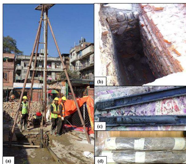
Figure 2. Pashupati location on December 10, 2017 (a) drilling operations, (b) removal of cultural materials (c) extracted disturbed sample and (d) undisturbed soil samples
