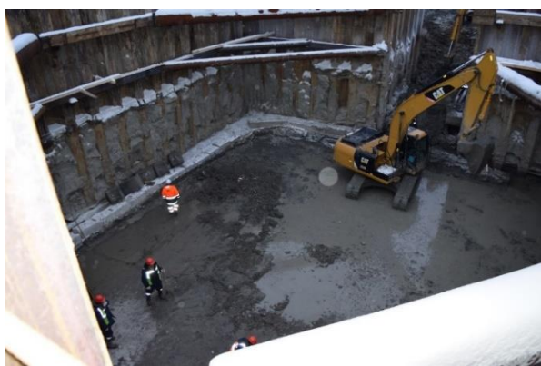
Figure 1. Flooding of the pit due to insufficient depth of GWC
