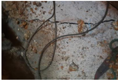
Figure 8. Structural failure of test segment during load test
