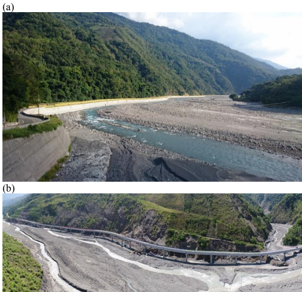
Figure 6. Figure 6-(a). The road alignment was adjusted at the northern end of this section, and several unstable slope units were avoided by lifting the road embankment closer to the river. Figure 6-(b). The viaduct form was selected at the confluence of tributaries to avoid the attack of debris flow. The mid-term road was completed in 2017. After several typhoons and heavy rainfall events in recent years, the road has survived safely.
