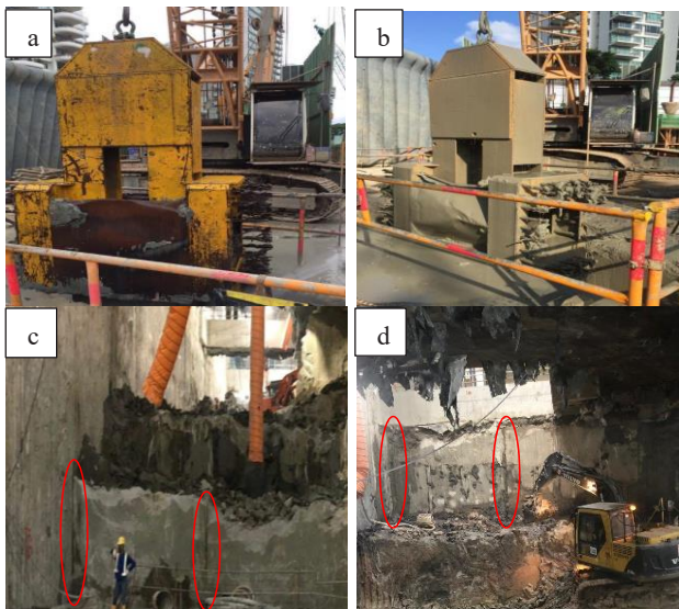
Figure 1 (a) & (b): Cleaning of diaphragm wall-cross wall joints using steel brush; (c) & (d): Diaphragm wall-Cross wall and Cross wall-Cross wall joints exposed during excavation
