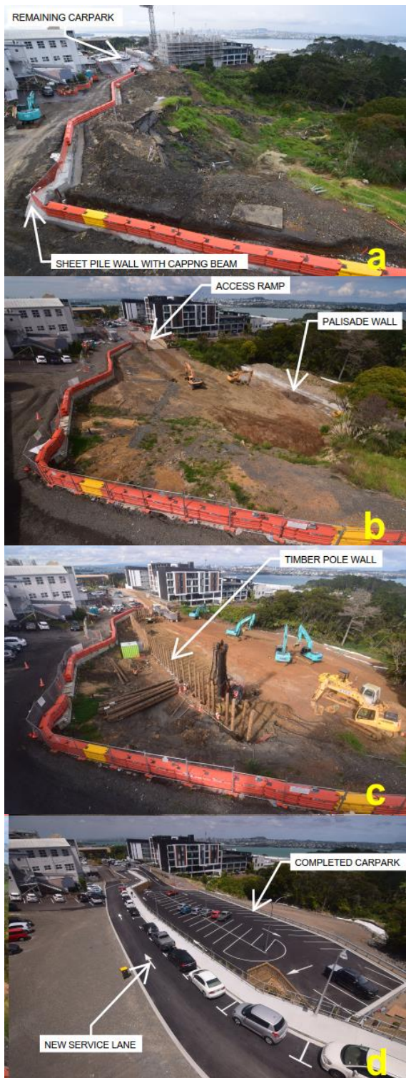
Figure 9. Photos of site from time-lapse camera: a) 28 June 2018 – Phase 1, prior to earthworks, b) 3 March 2019 – Phase 2, palisade wall completion, c) 5 July 2019 – Phase 2, fill 90% complete, timber pole wall construction, d) 22 November 2019 – carpark completion.
