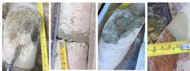
Figure 5. Areas of grout identified within boreholes drilled below the toe of the diaphragm wall
