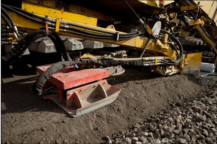
Figure 1. Plate compactor WBB 530 of the AHM 800-R during compaction of the FPL. Source: P&T
