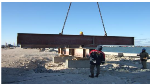
Figure 3. Support structure or platform for perception reaction forces (the system beams with anchor piles).
