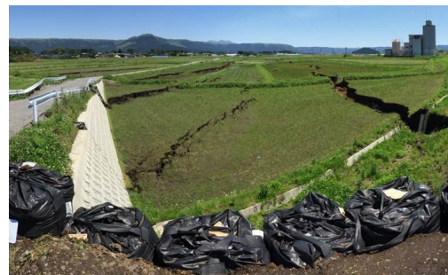
Figure 1. The depression zone as viewed by GEER from a local bridge.
