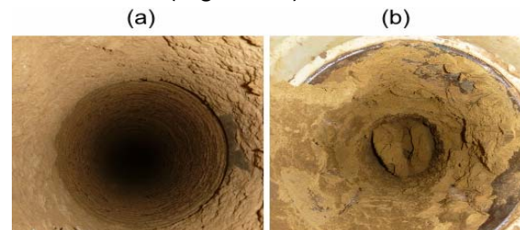
Figure 14: Free 10'' suction tube (a), clogged suction tube (b)
