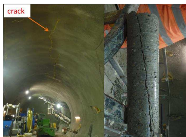
Figure 2. (left) Location of the longitudinal crack at the crown (right) depth of the crack
