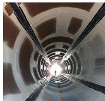
Figure 1. Inside view of an instrumented monopile, black lines are optical fibres on which the FBGs are mounted at different depths.
