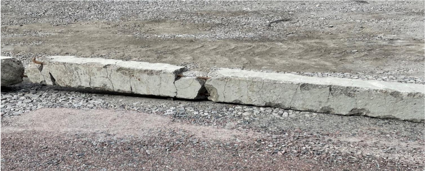
Figure 1. An example of structural failure in a concrete pile
