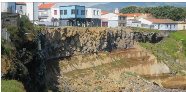
Figure 3. The cliff after the instability of April 7.
