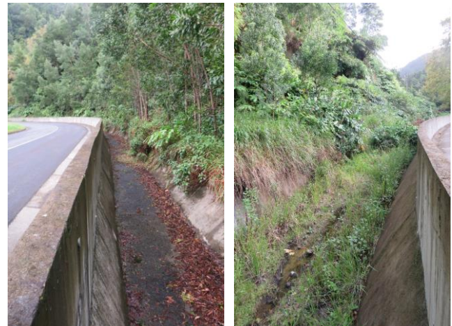
Figure 5. Site no. 5 – Retaining wall with ditch (on the left). Site no. 7 – No maintenance (on the right).
