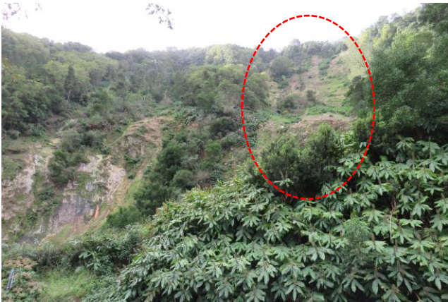
Figure 7. Geomorphological instability, of debris avalanche type, on the slope adjacent to the semi-tunnel.
