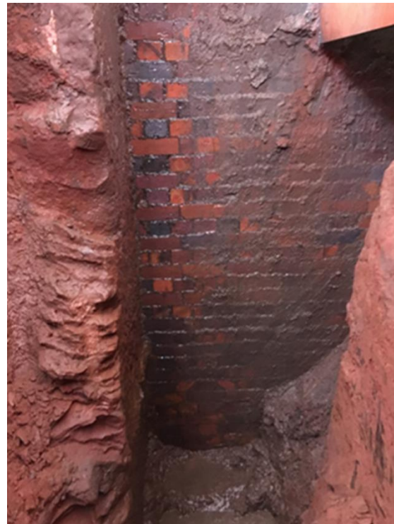
Figure 3. Trial trench perpendicular to pier at Arch 23 illustrating the quality of the rock and bedding.
