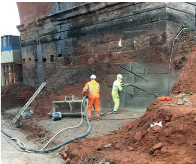
Figure 5. Placing hard facing to the initial working bay below the north footing of arch 23.
