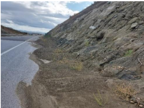
Figure 1. Erosion on the slopes between the 2 extreme rainfall events on May 29, 2022.
