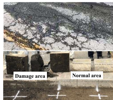
Figure 1. Early deterioration of asphalt pavement.
