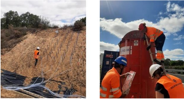
Figure 3. Installation of the injection pipes (left) and mixer used to prepare the bacteria and feeding fluids (right).
