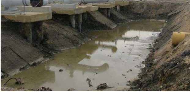
Figure 2. Excavation with unstable sloping sides.
