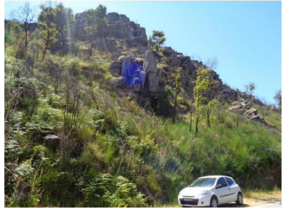
Figure 1. View of the slope showing the heavily fractured rock mass at a high elevation with potential for instability.
