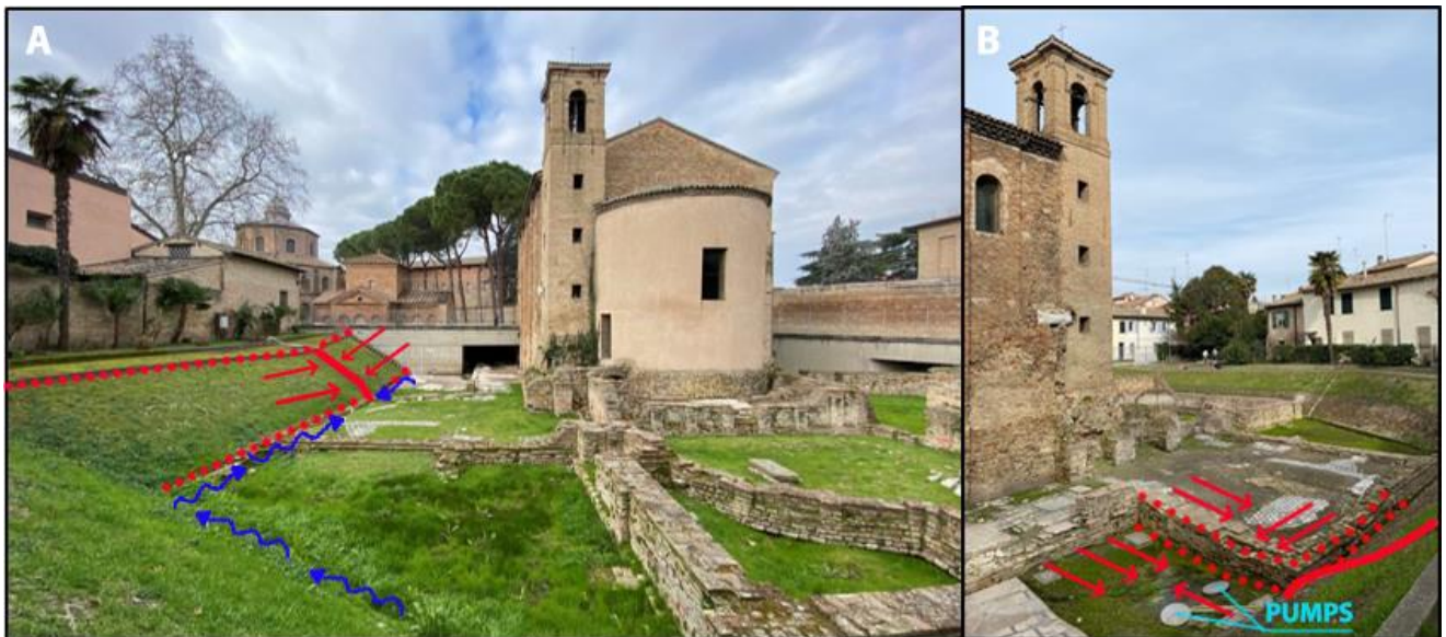
Figure 3. Pictures highlighting the different types of deterioration to the masonry structures and to the earthen slope of the basin, caused in time by the operating drainage system.
