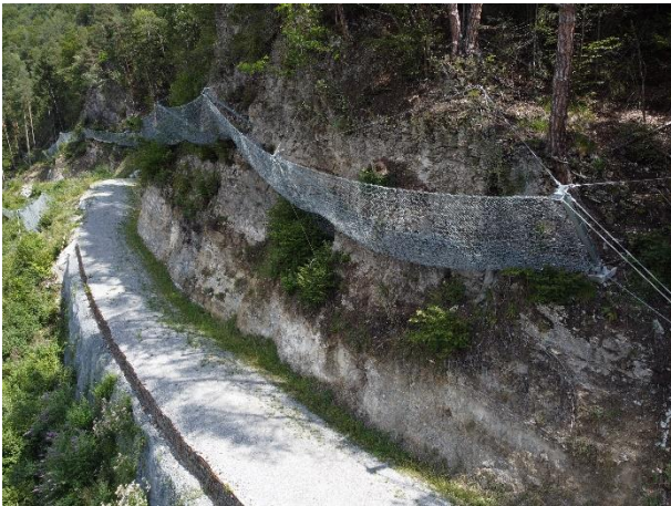
Figure 1. Rockfall protection net next to a support road of a railway line.
