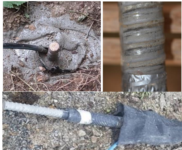
Figure 2. Types of corrosion protection, top left: grout cover protection (GCP), top right: zinc corrosion protection (ZCP) and double corrosion protection (DCP).
