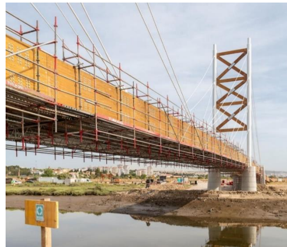
Figure 10. Bridge view just before the YWD, August 2023 with the deck being reinforced for the pope's car crossing.
