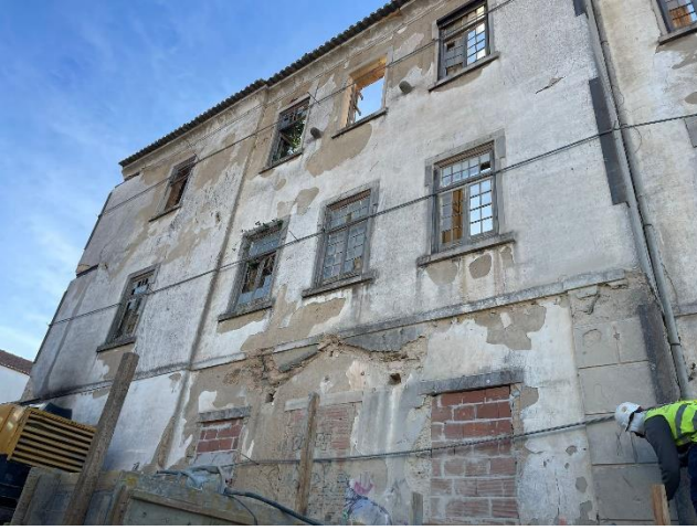
Figure 4. Prior facade retention works, involving the installation of steel angles and steel tie rods per floor.
